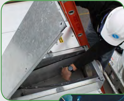
Inlet strainer inspection for Series 1500
